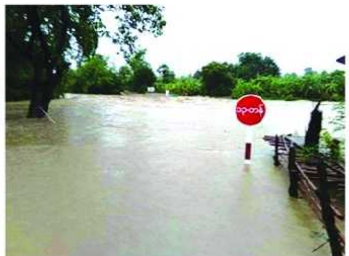
Submersible bridge will be under water a few times a year in rainy season.
